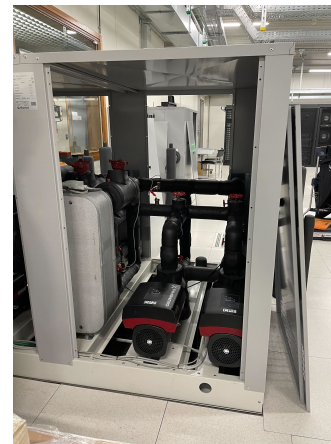
Pumps in HPC room dedicated for Hortense cooling circuit
