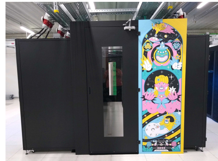
Front view of Hortense Right block: phase 1 (Rome) Left block: phase 2 (Milan)
